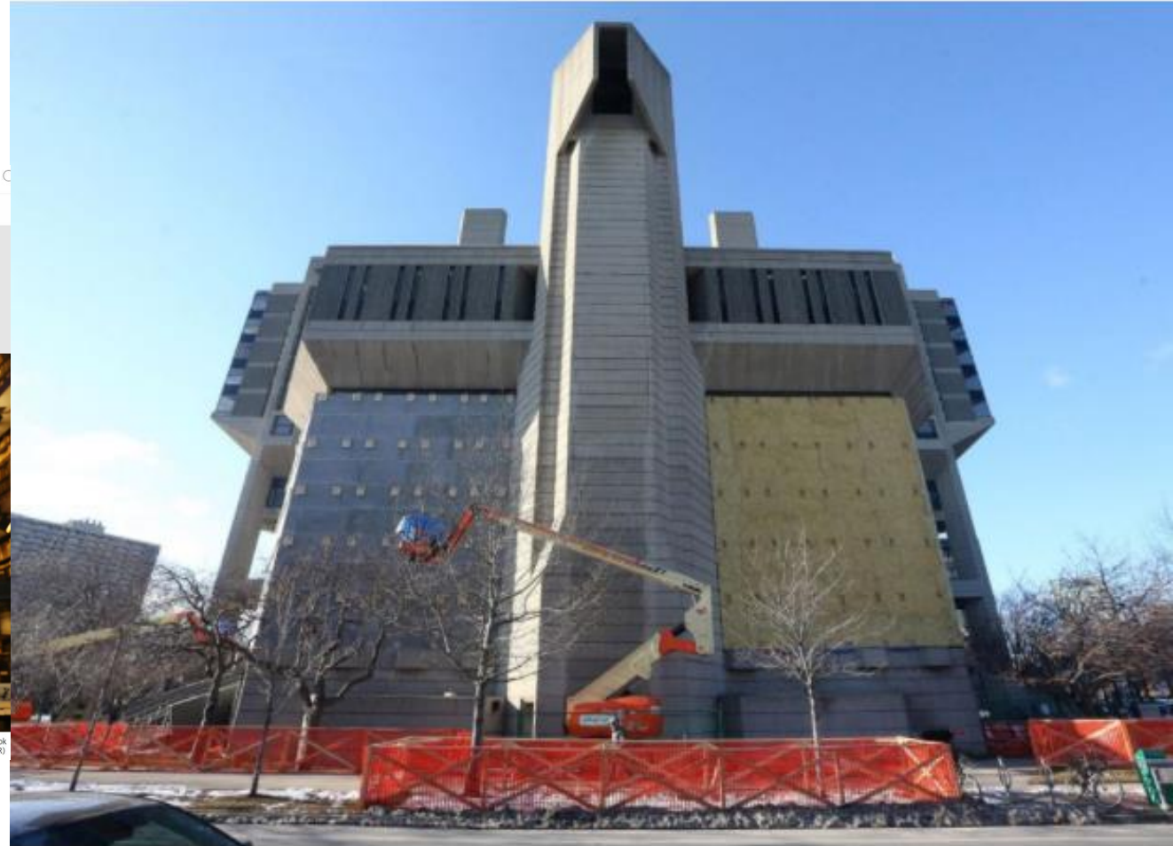
A group of first year engineers came up with an idea to insulate the outside of the library with concrete sheeting over spray foam. (STEVE RUSSELL / TORONTO STAR)
